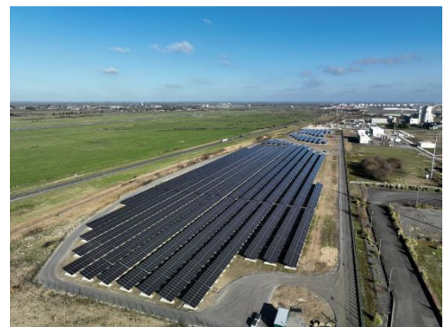
Sited to the east and to the north of the LNG terminal, the photovoltaic power plant operated by Engie Green.
