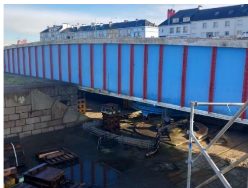
Refurbishment work on the swing bridge of the south lock, in Saint Nazaire.
