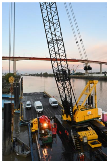
The Aloès crane barge, here being used for the refurbishment of the dolphins of the Cheviré ro-ro berth.
